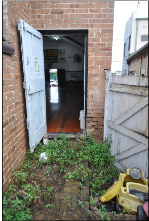
Figure 23. View of north western corner of original building showing original door and significantly eroded mortar and collapsing brickwork.
