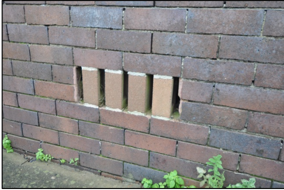
Figure 19. Unsympathetic ad-hoc ventilation at sub floor level.
